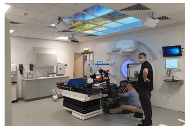
Oldham linac installation
