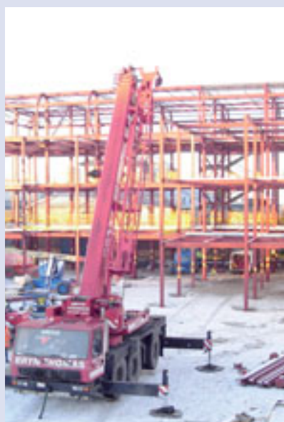
▲ Under construction: Half of the steelwork is now in place for the Oldham centre.
